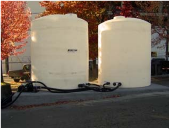
10,000 Gallon Salt Brine Storage Tank
