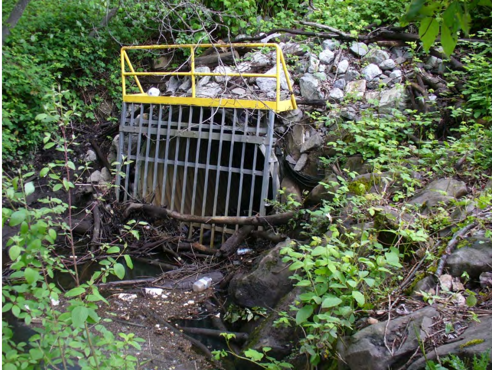
Photo 5. Trash rack and debris at the inlet of the 66th Avenue S culvert.
