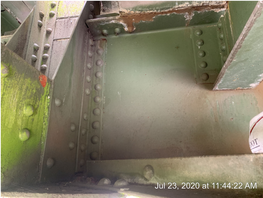
Inspection Photo 7 – Rust at Top Flange of Fracture Critical Floor Beams
