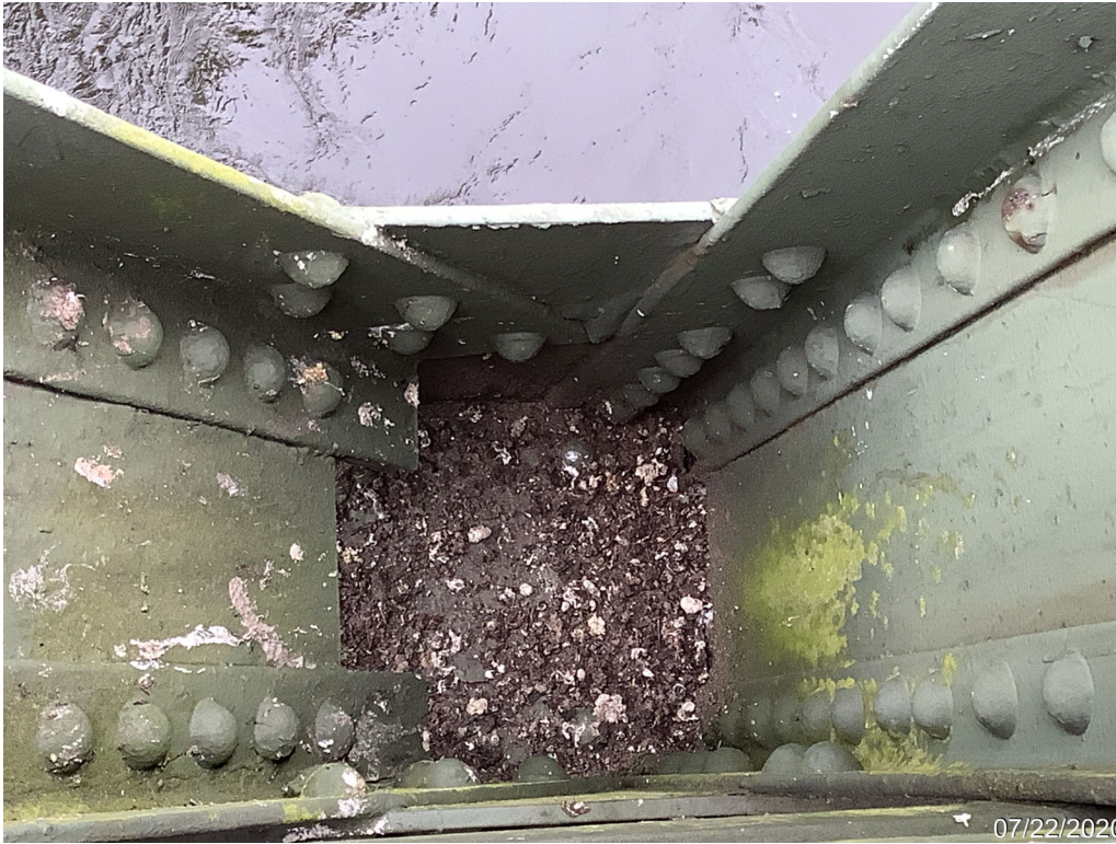
Inspection Photo 3 – Lower Connections with Horizontal Gussets Retain Moisture and Guano
