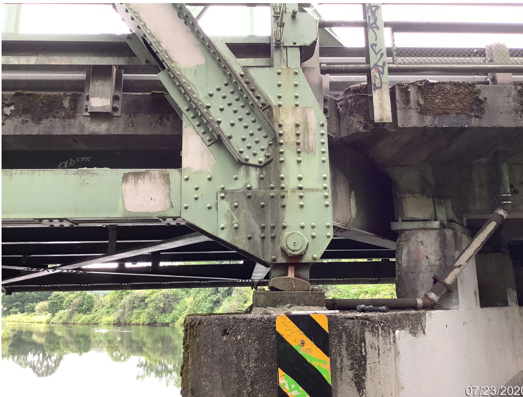
Inspection Photo 4 – Frozen Truss Bearings Induce Additional Stresses on the Trusses
