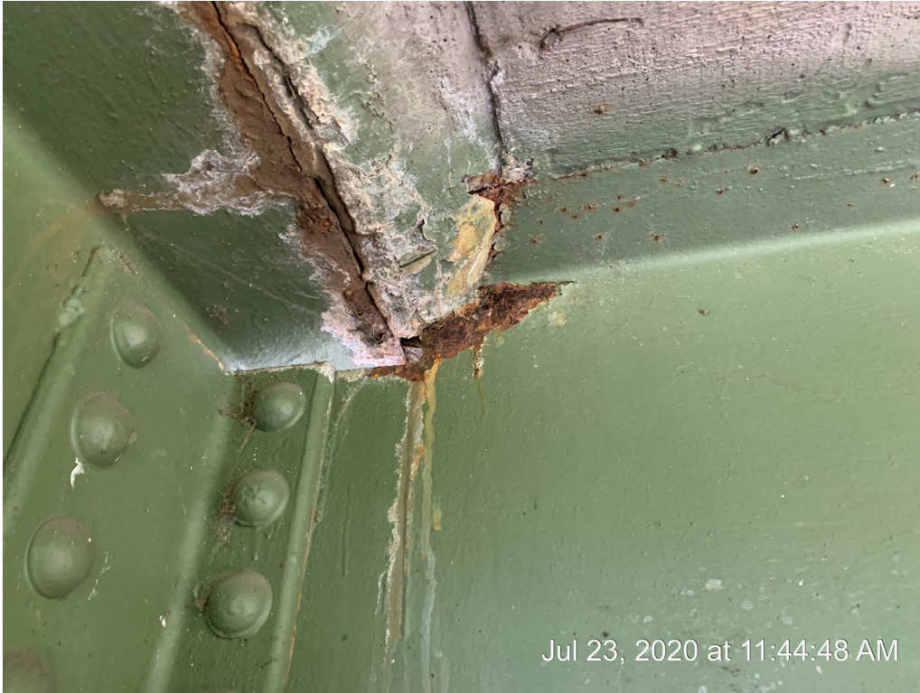
Inspection Photo 8 – Moisture from Deck Penetrating and Corroding Top Flange of Stringers
