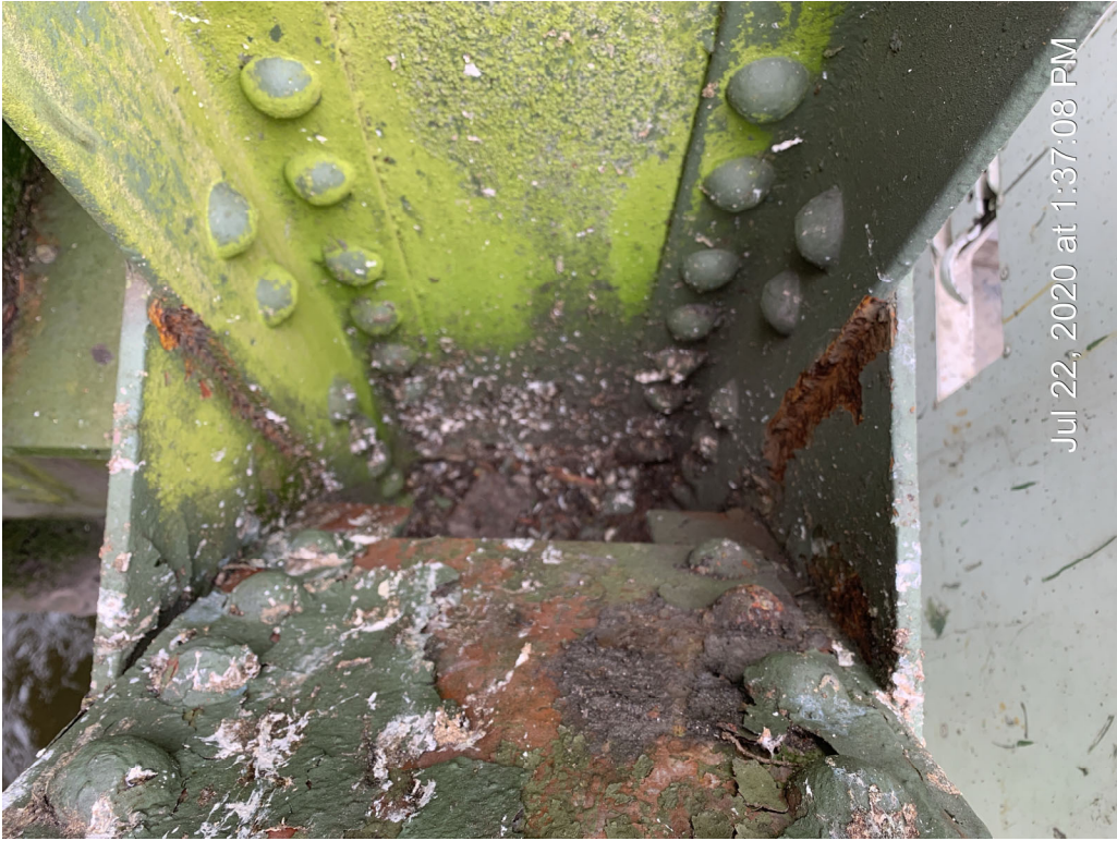
Inspection Photo 6 – Rust and Guano at Truss Bottom Chord
