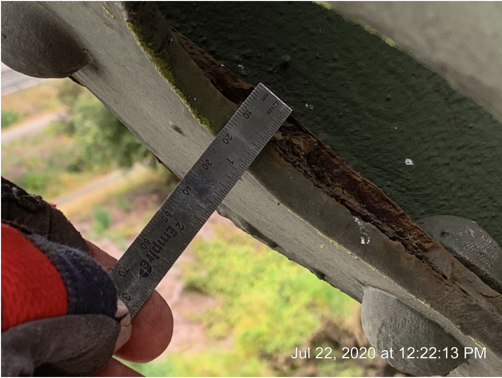
Inspection Photo 5 – Pack Rust is Distorting some Connections
