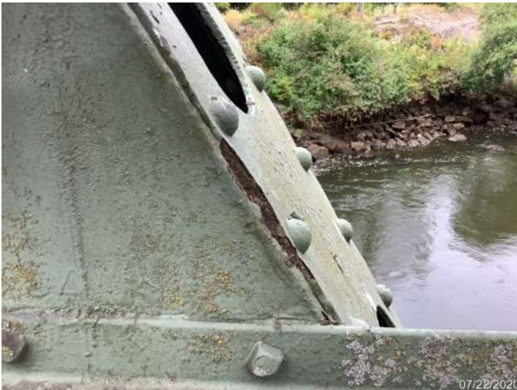
Photograph 6: Area of pack rust on the diagonal bridge beam
