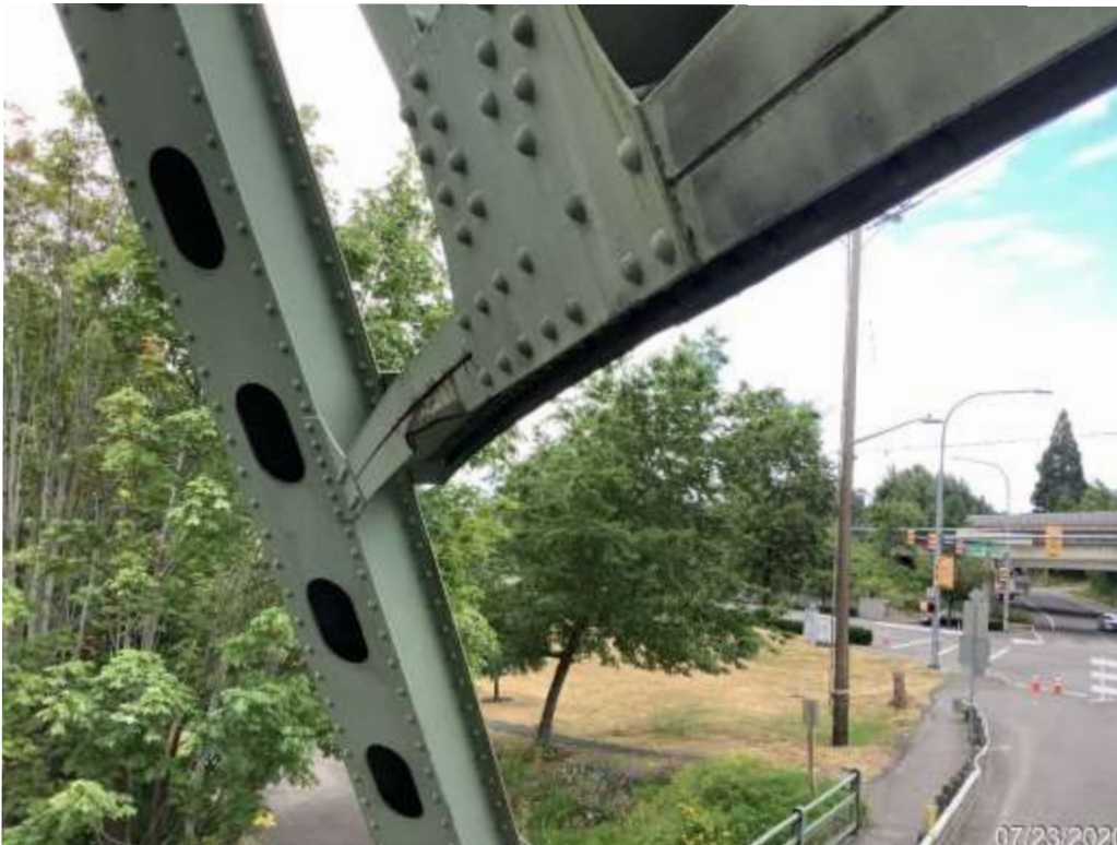
Photograph 8: Impact damage due to truck collision on the south approach
