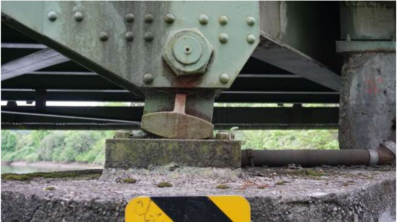
Photograph 3: Frozen bearings on the bridge not allowing bridge to adjust for temperature
