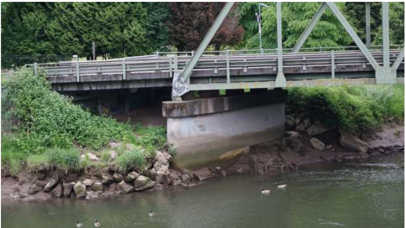
Photograph 4: Washed away embankment material on the north pier
