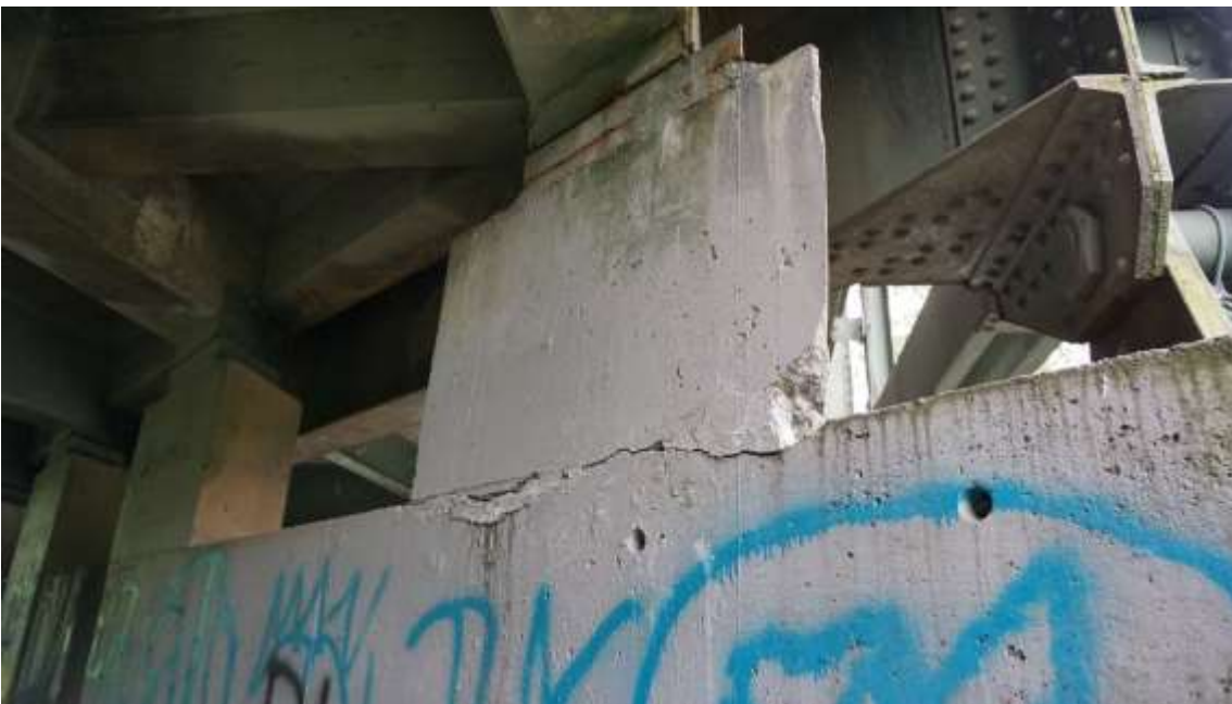
Photograph 2: Crack in the concrete pier on the northside of the river
