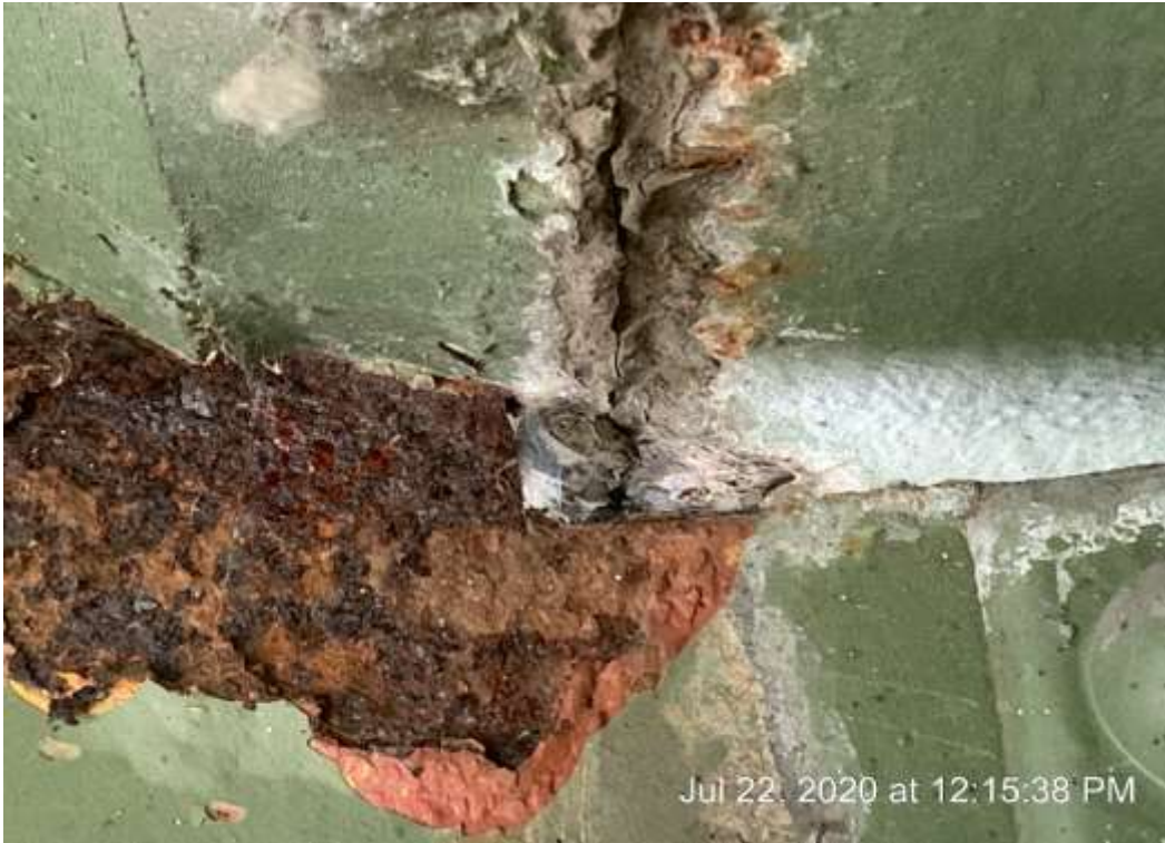
Photograph 5: Typical area of rust on critical areas of the bridge
