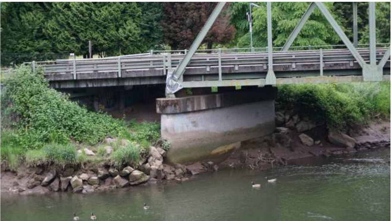
Photograph 4: Washed away embankment material on the north pier
