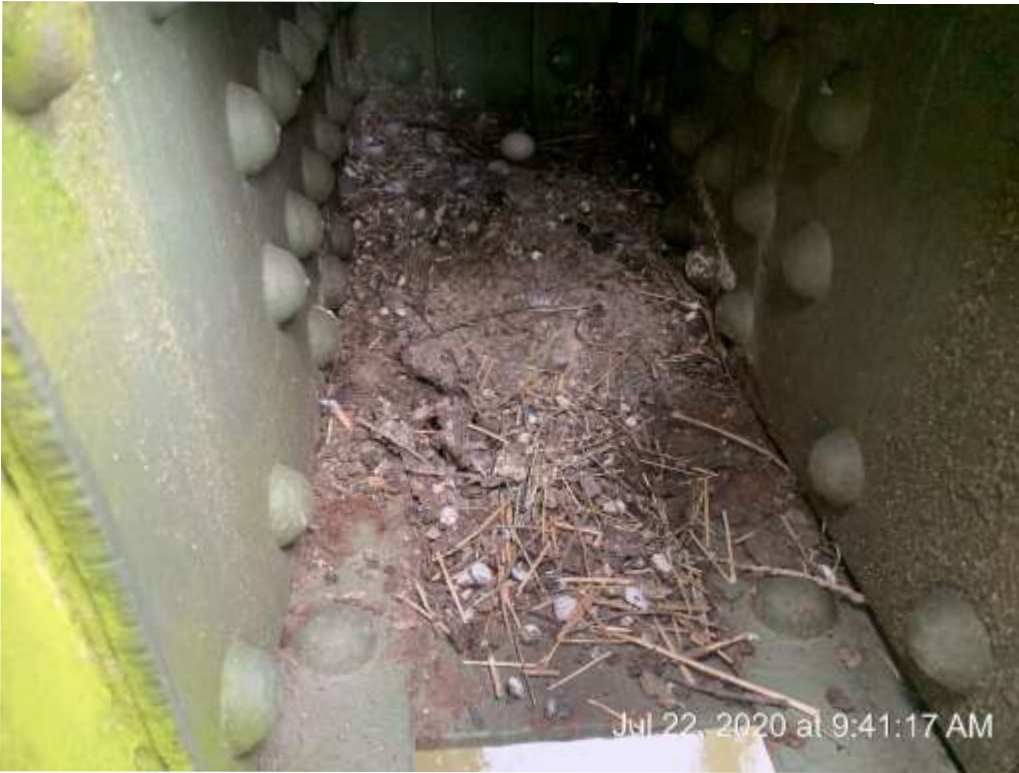
Photograph 7: Typical accumulation of pigeon guano causing corrosion
