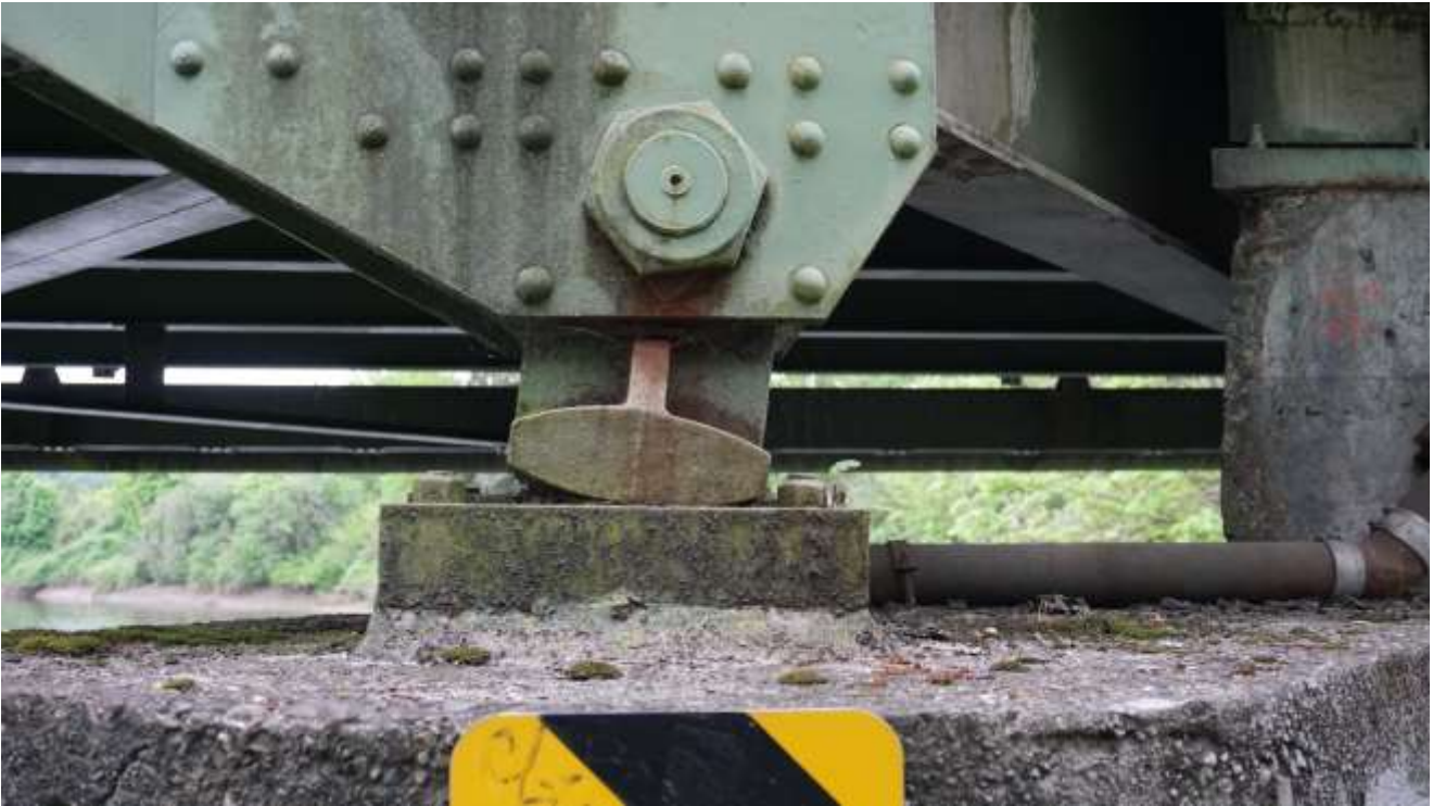
Photograph 3: Frozen bearings on the bridge not allowing bridge to adjust for temperature
