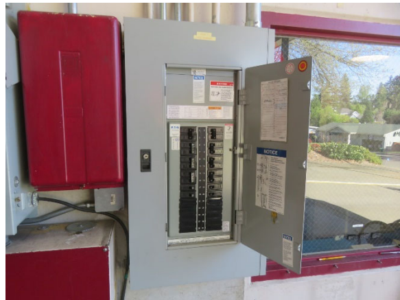
One of Several Electrical Service Panels
