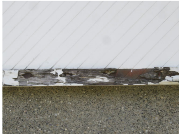
Rot in the Trim of the North Side of the Building
