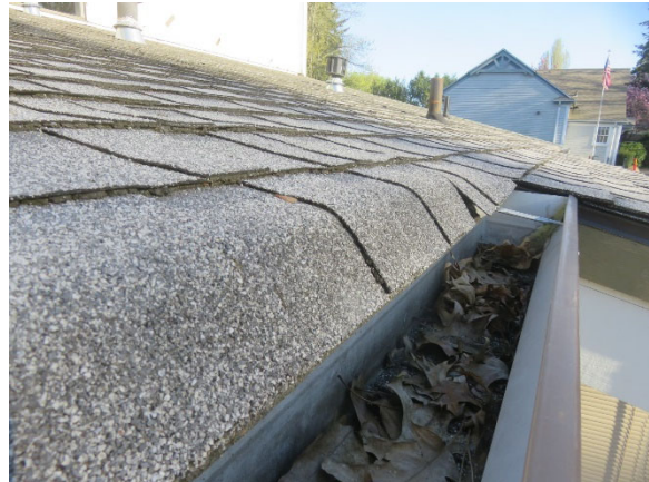
Shingles Bent into Gutter on Lower Roof of the Building
