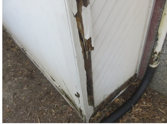
Rot Present on the West Side of the Building
