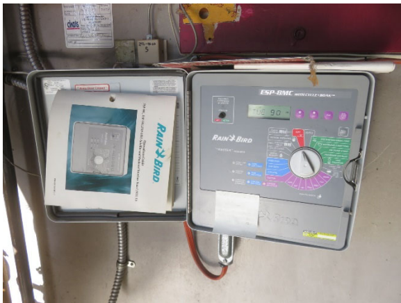
Irrigation System Control Panel
