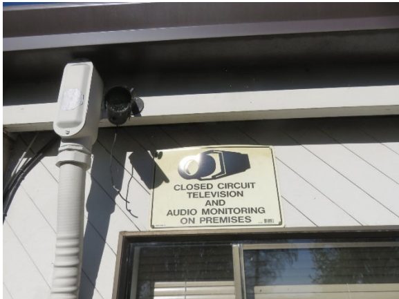
Old Surveillance Camera
