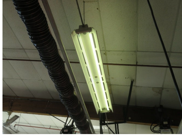
Typical Hanging Fluorescent Light in the Engine Garage Bays
