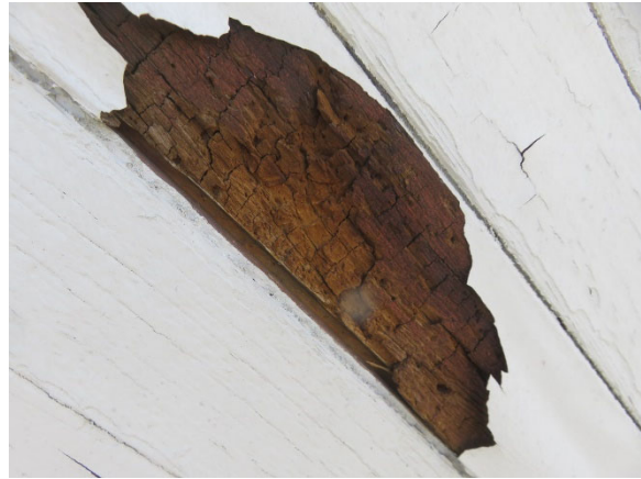
Rot in the Siding of the West Side of the Tower
