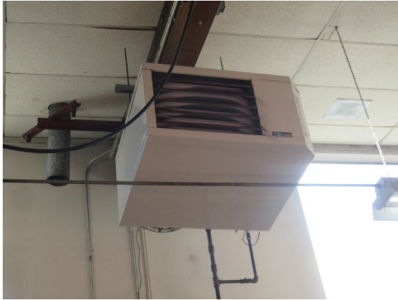
Hanging Reznor Furnace
