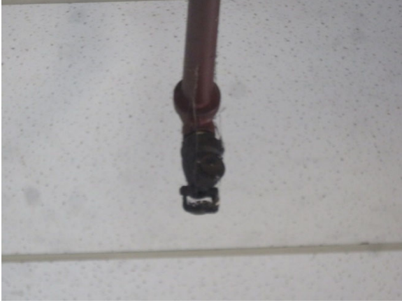
Typical Fire Suppression Sprinkler
