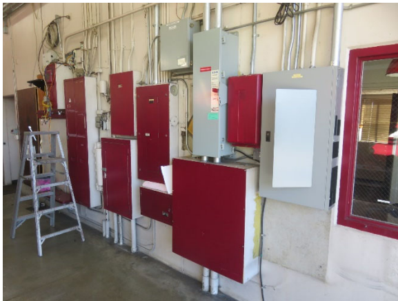
Electrical Service Panels
