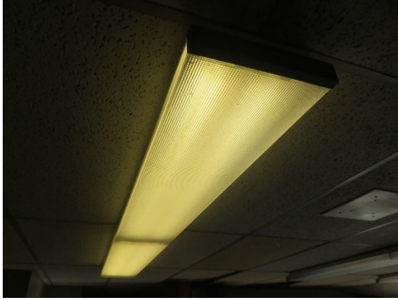
Typical Hanging Fluorescent Light in the Office/Sleeping Quarters
