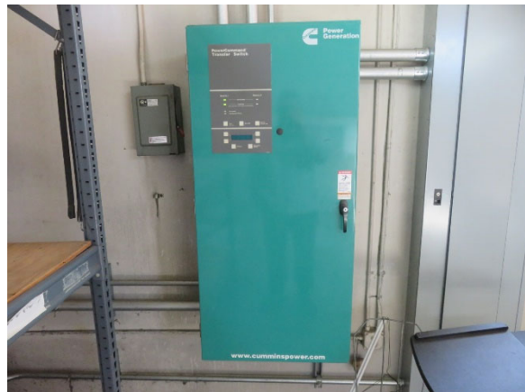
Generator Transfer Switch
