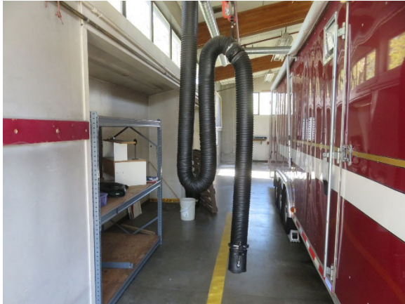
Exhaust Capture Hoses
