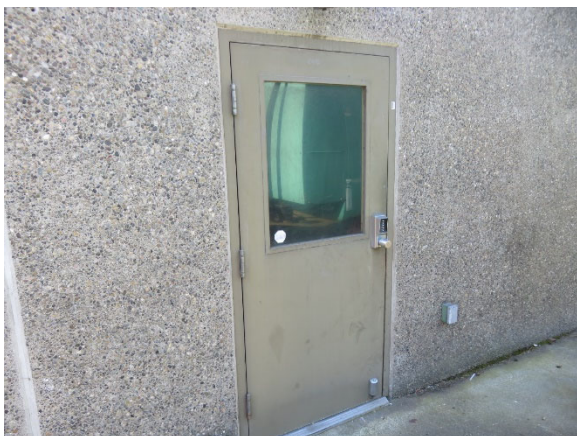
Metal Service Door with a Window
