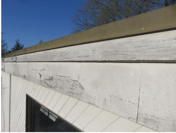
Rotten Trim of the Clerestory
