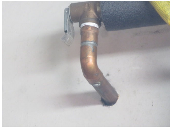
Typical Copper Supply Piping
