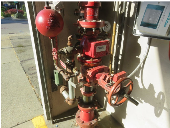
Fire Suppression System Manifold
