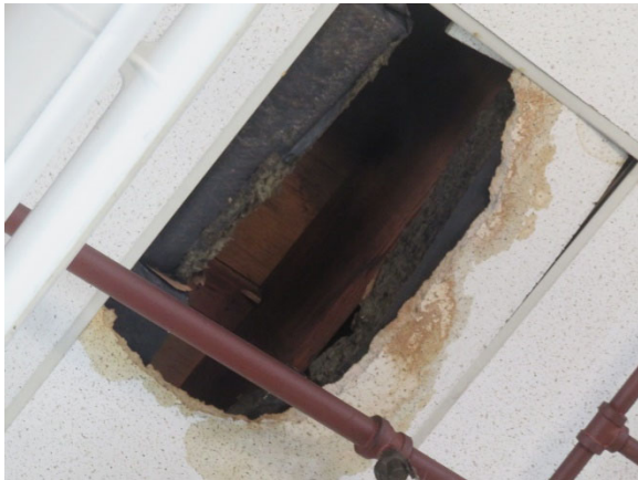
Wood Rafters Visible in the Damaged Ceiling
