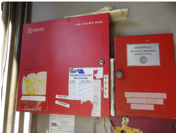
Fire Alarm Control Panel
