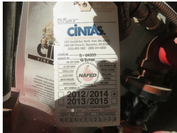
Fire Suppression System Formerly Maintained by Cintas
