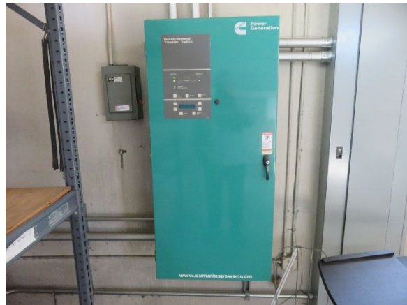
Generator Transfer Switch
