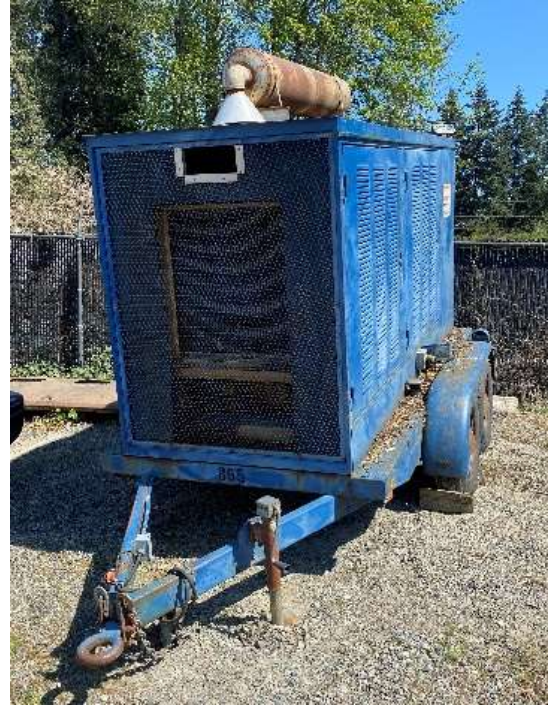
Unit 1865, 1983 Kohler 80KW generator trailer, 1,013 hours. Plate: D33858. S/N: 144079. Estimated value: $2,300
