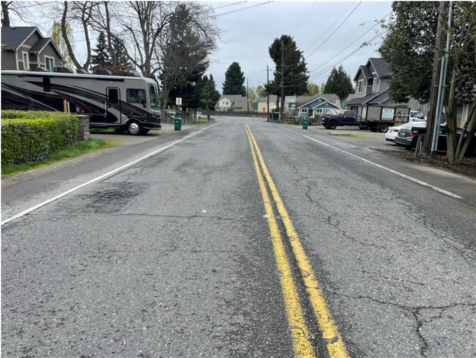
Cracking on roadway, missing RPMs, and faded paint on 50 th Pl nearing the S 124 th intersection facing North
