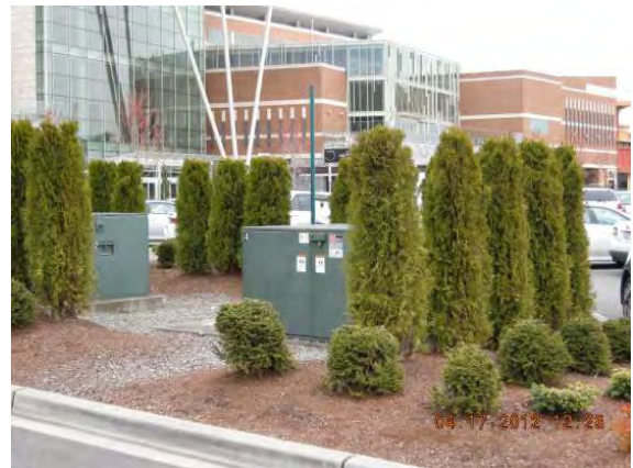
Figure 18-48: Using evergreen landscaping to screen utilities
