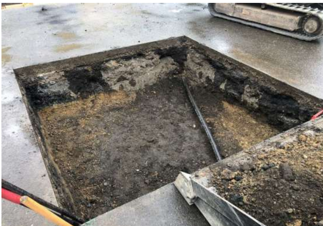
EXISTING WATER LINE DISCOVERY IN COMPRESSOR BUILDING FOOTING ZONE
